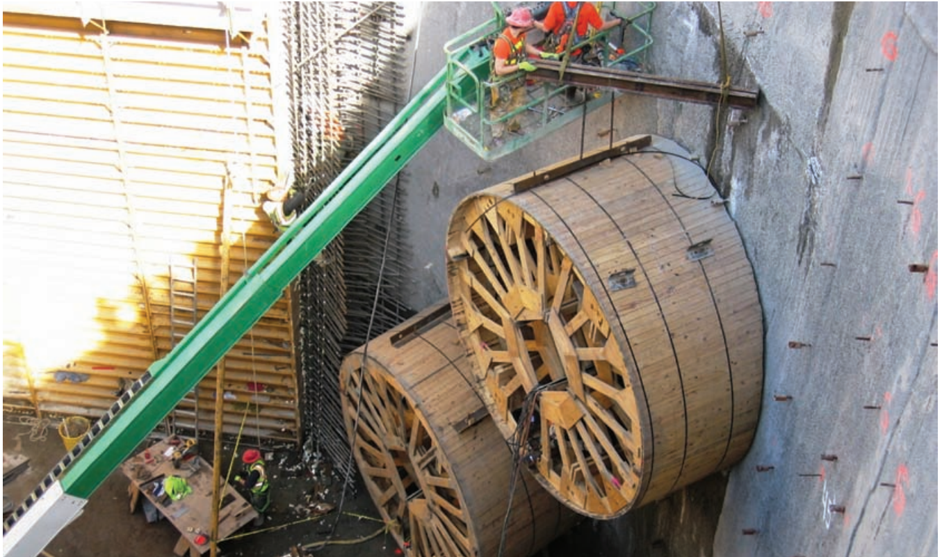
The final lining blockout forms for the influent structure to the influent pump station connector tunnels at the North Creek Portal influent structure.
